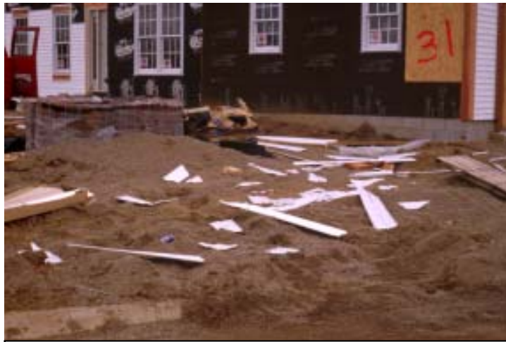
Figure 1. Remove all construction debris, pea gravel, concrete spoils, etc., prior to establishment to minimize future turf problems.
