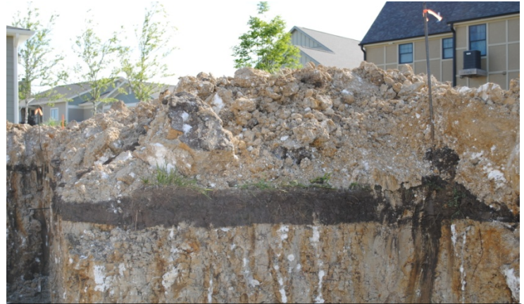
Figure 2. Stockpile topsoil prior to establishing rough grade and then return topsoil to the site, preferably establishing four inches of topsoil over subsoil.
