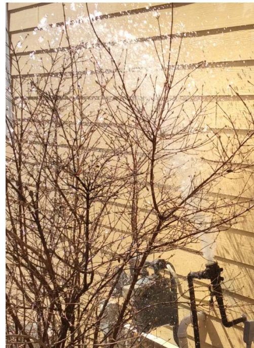
Water 'geyser' from a frozen backflow preventer
